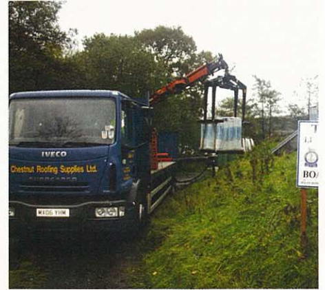
The products were delivered by one of IKO's customers, Chestnut Roofing & Building Supplies, in January 2011
