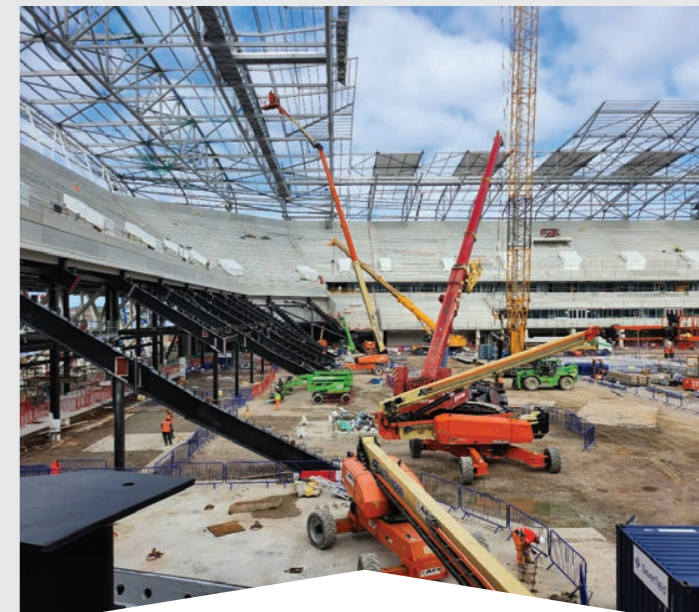
The 13-row concrete seating of the stadium is now in place, covered by a 45m high cantilevered roof structure.
