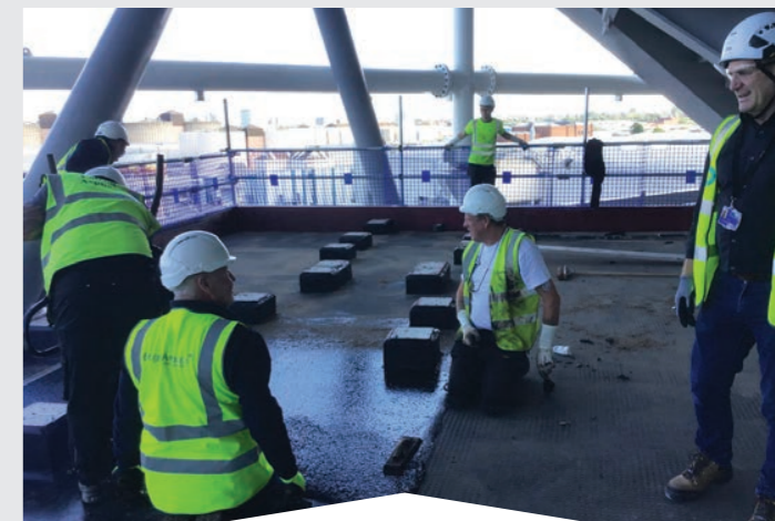
Tony is visiting the Everton site every week to check on progress and quality. As a time-served mastic asphalt roofer who worked on the tools for 15 years, his knowledge comes from practical experience as well as from his years in management.
