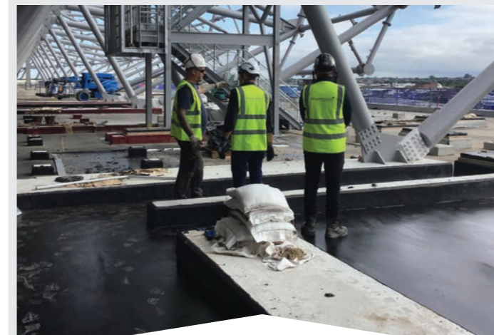
The mastic asphalt roof on the stadium’s east side is well underway. The roof consists of three layers: an isolation layer is laid on the concrete deck before the first 10mm layer of mastic asphalt is applied. A final 10mm top layer is finished with a white, solar-reflective coating to help minimise the roof-temperature and thermal movement across the stadium’s roofs.
