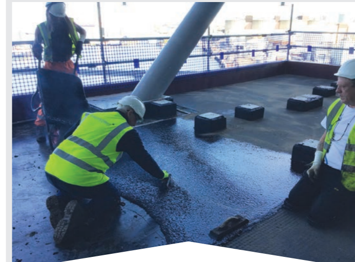
The molten mastic asphalt is wheelbarrowed from the nearby hot boiler to the stadium’s west side roof area where it’s poured. The waiting roofers have to work quickly before the 180°C asphalt cools. It’s a highly-skilled job to ensure the asphalt is laid level, to the correct depth and the joints are watertight.
